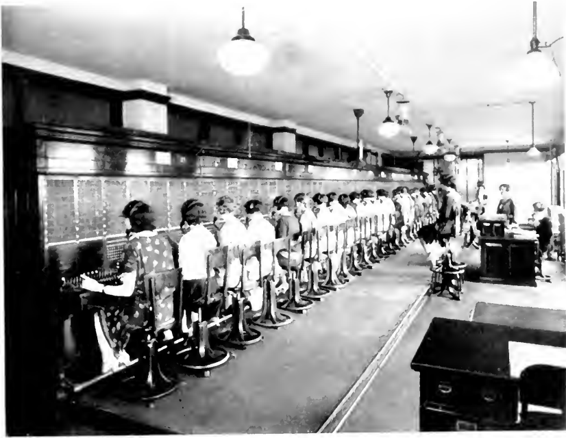
FIGURE 2. THE LOCAL SWITCHBOARD IN ANDERSON AS IT WAS BEFORE THE FIRE.
